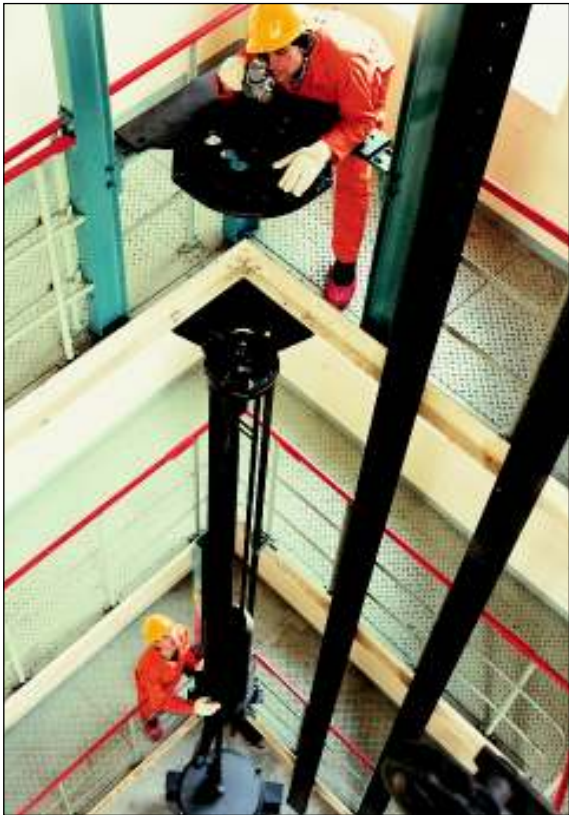
Alignment of a refuelling system in the nuclear power industry.
